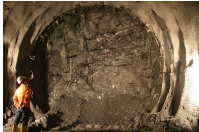
Front face of Exploratory Tunnel in Mules Fault Line (schist and micaschist, phyllite).
